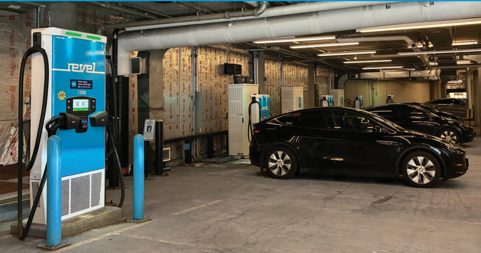
Jackson Avenue Charging Hub, Long Island City, NY
