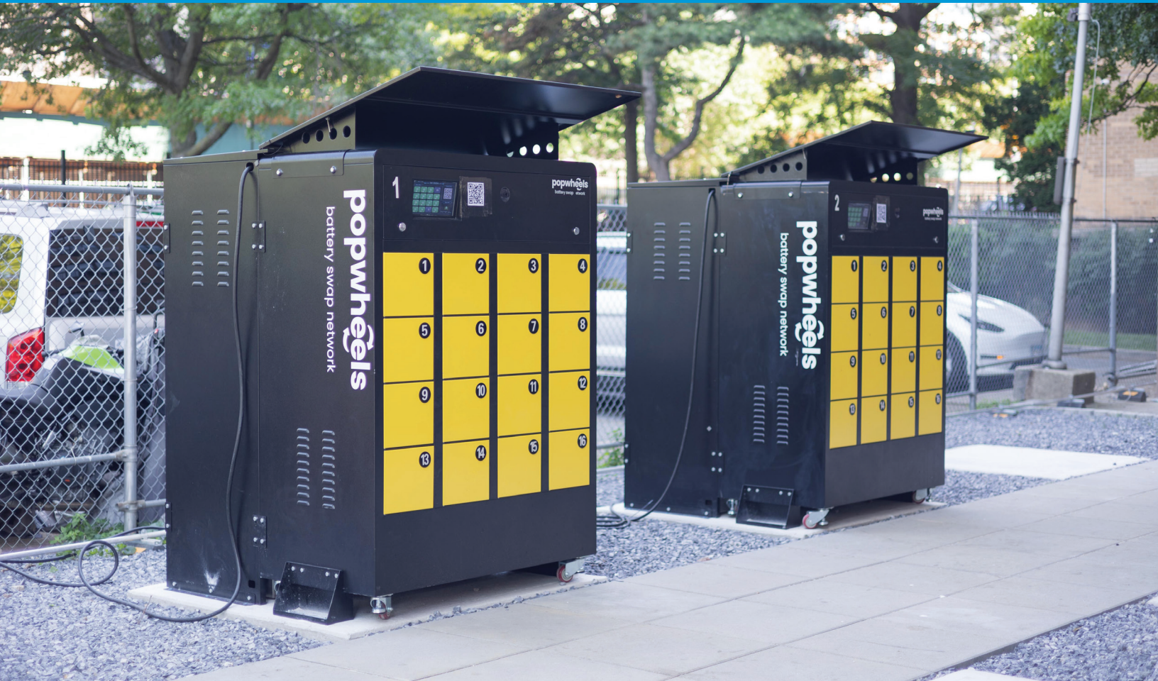
E-Bike Battery Charging Cabinets, Brooklyn, NY
