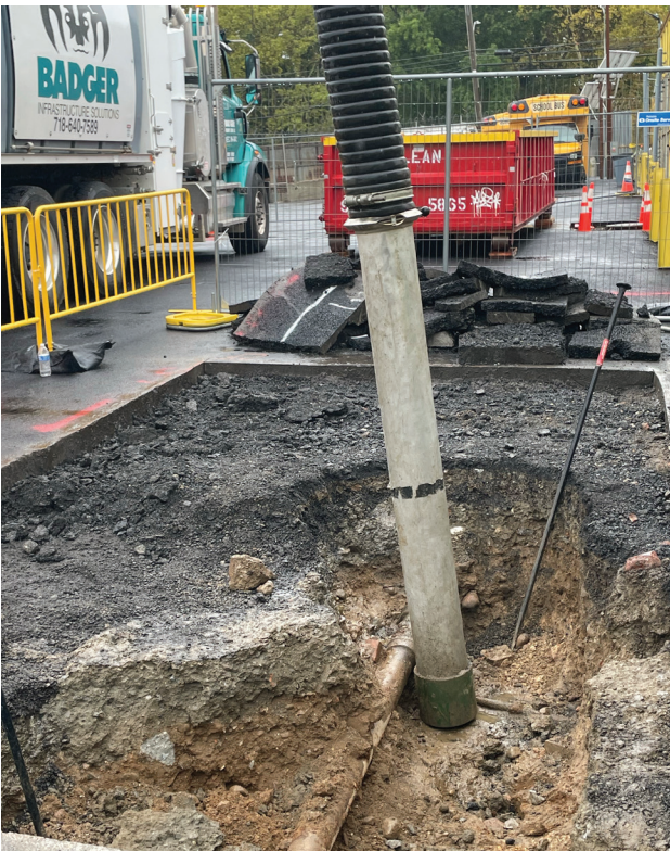
Underground Trenching Obstructions
