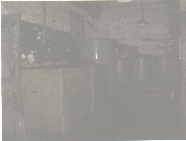
Miscellaneous tanks located in the tank room.
