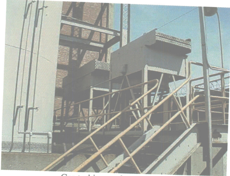
Gas turbine coolers, typical.
