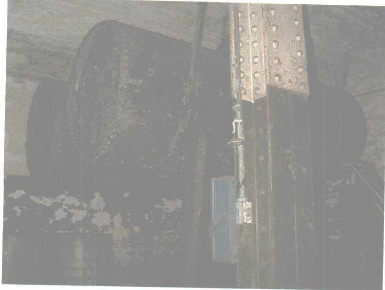
Overhead tanks in tank room.
