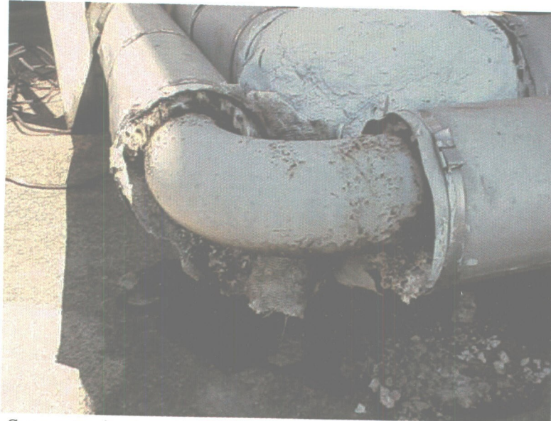
Suspect asbestos containing material located by the former 40,000-gallon capacity kerosene storage tanks.
