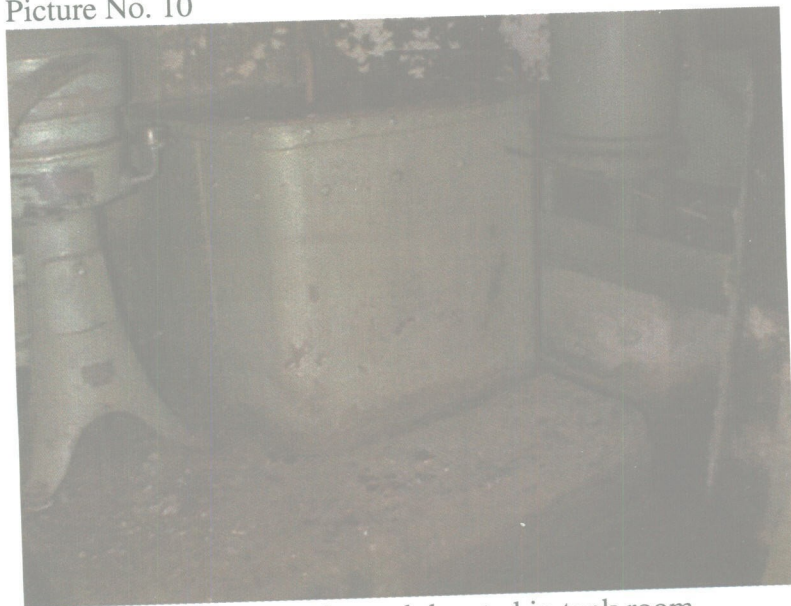
58-gallon capacity tank located in tank room.
