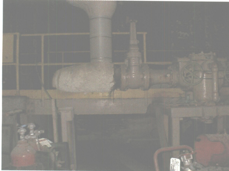
Suspect asbestos containing material located in the Williamsburgh Turbine House.
