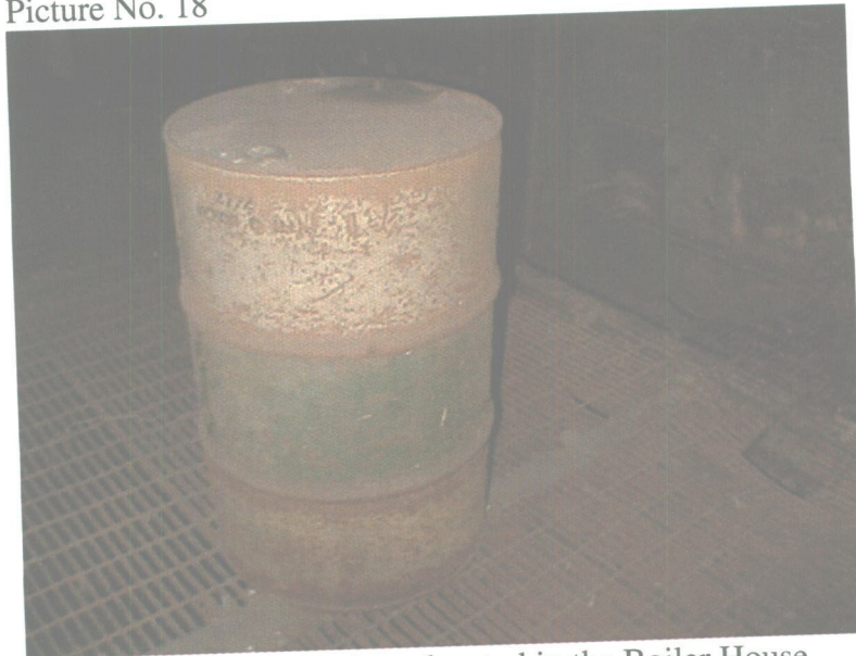
55-gallon capacity drum located in the Boiler House.
