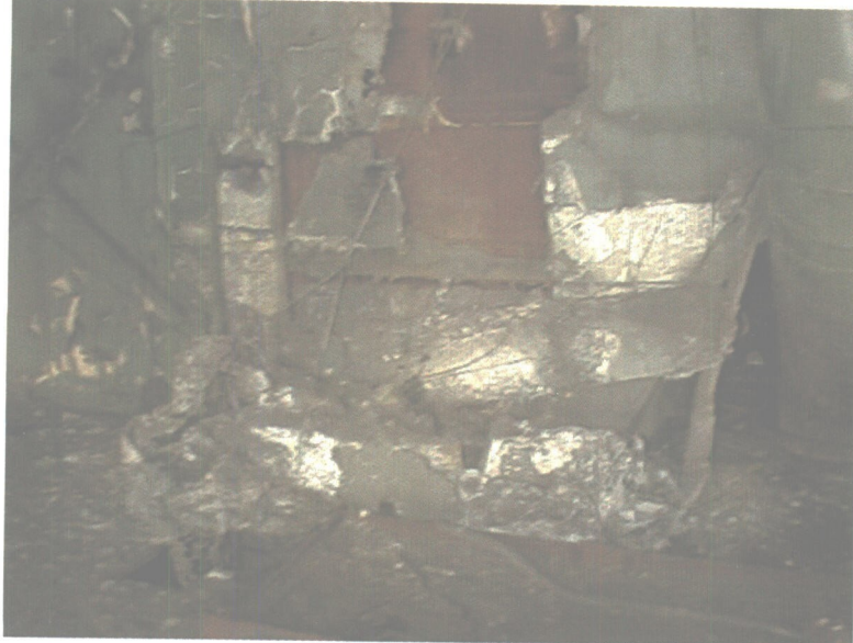
Suspect asbestos containing material located within the Boiler House.
