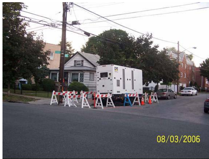
Figure 4-10: Mobile Generator Set Up in LIC
