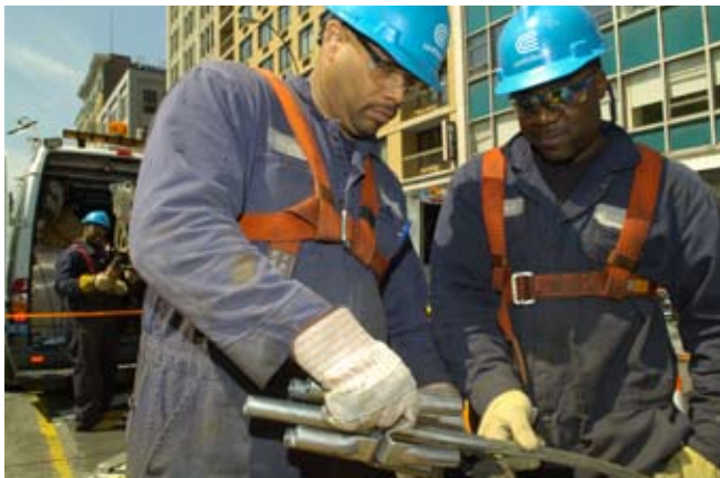
Skilled splicers maintain and reinforce the most reliable electricity delivery system in the nation.
