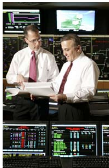
A state-of-the-art control center ensures that the natural gas transmission and delivery system can respond quickly and efficiently to systems needs, from the greatest to the smallest in the field.
