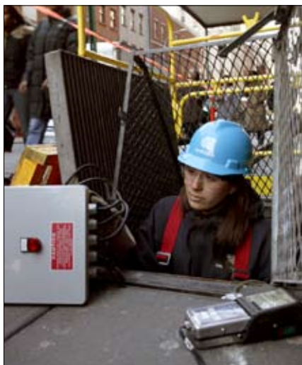
CECONY installs “oil minder” units in underground facilities and equipment that normally empty to sewers to prevent the release of oil to the environment.
