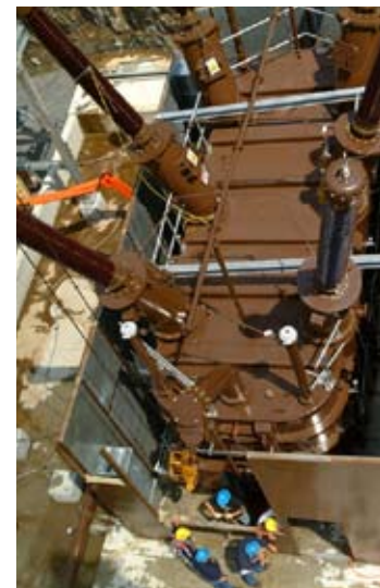
The installation of a new transformer at a major transmission substation in Westchester County helps ensure adequate power and continued reliability.
