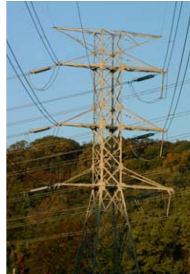
Transmission towers deliver electricity to Con Edison and Orange and Rockland customers.
