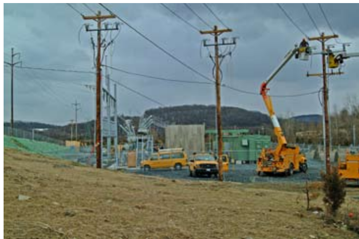
Orange and Rockland crews sharpen their skills at their state-of-the-art electric overhead school.
